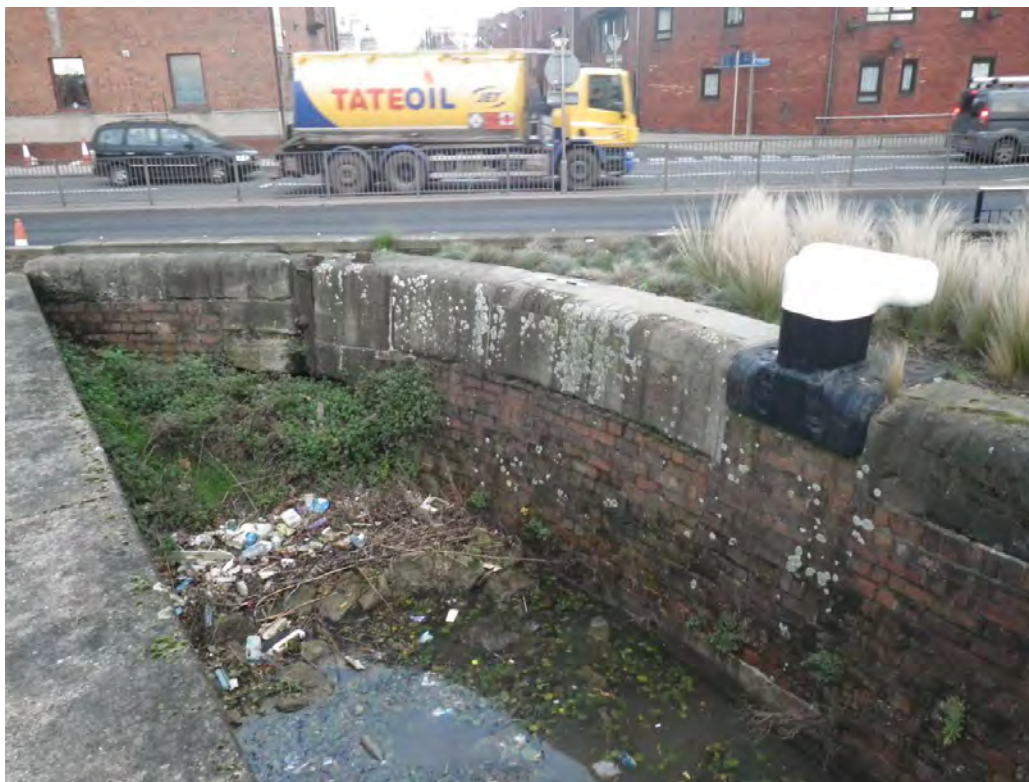
Plate 2: Dock wall (item 26), mooring post (item 5) and sluice gate (item 6), looking north-east
