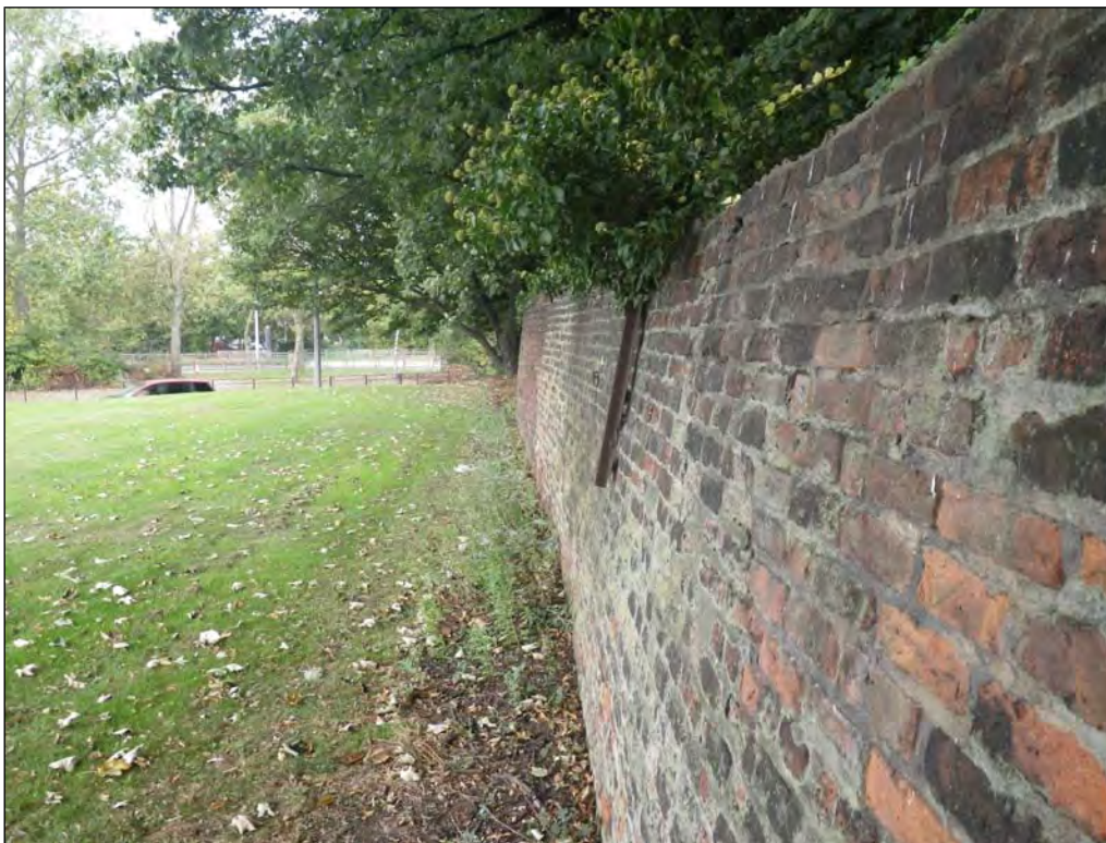
Plate 4: A view along the west wall, looking north and showing the pronounced lean to the central section of the wall
