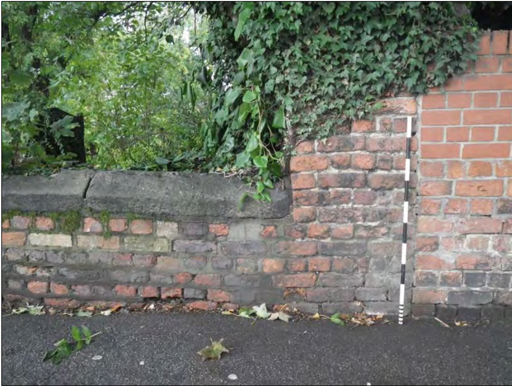
Plate 13: Pier at the junction of the west and the north walls (left of photograph). The relationship between the pier and the west wall was not observed due to vegetation coverage (1m scale)
