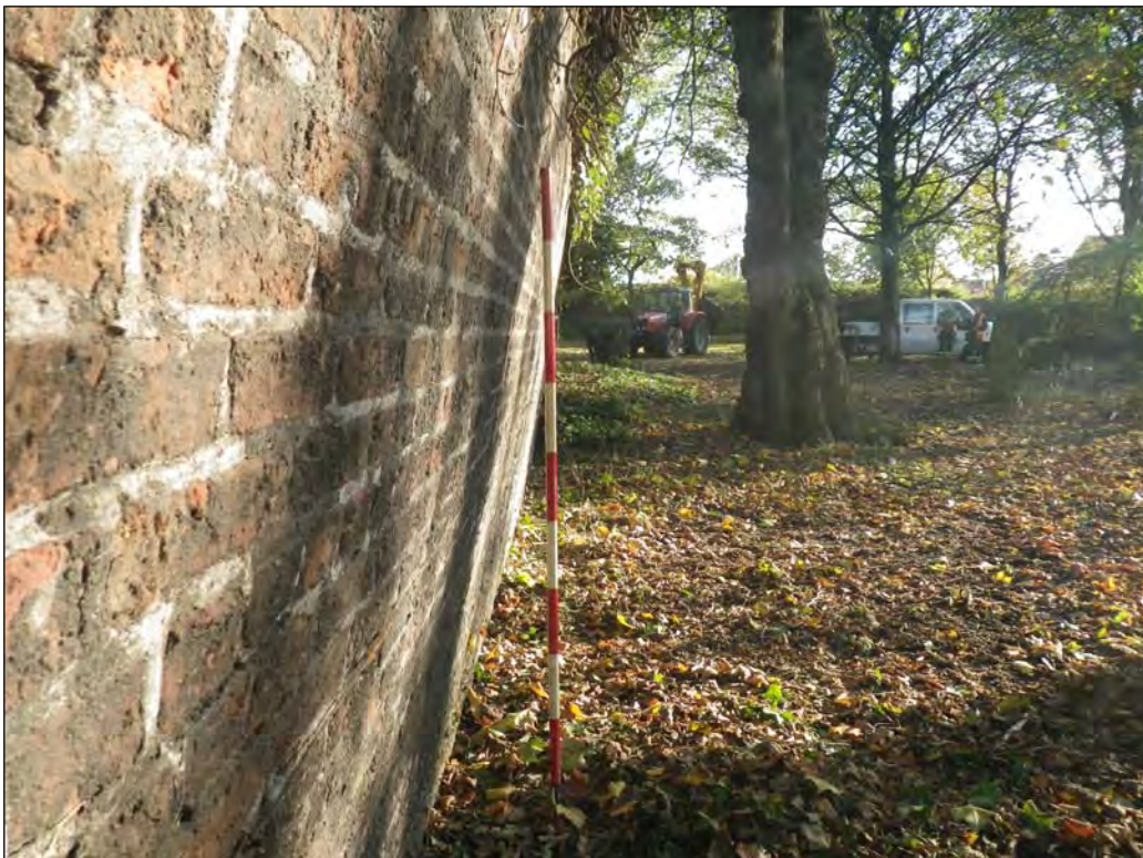
Plate 24: The pronounced lean on the western face of the gaol-yard wall
