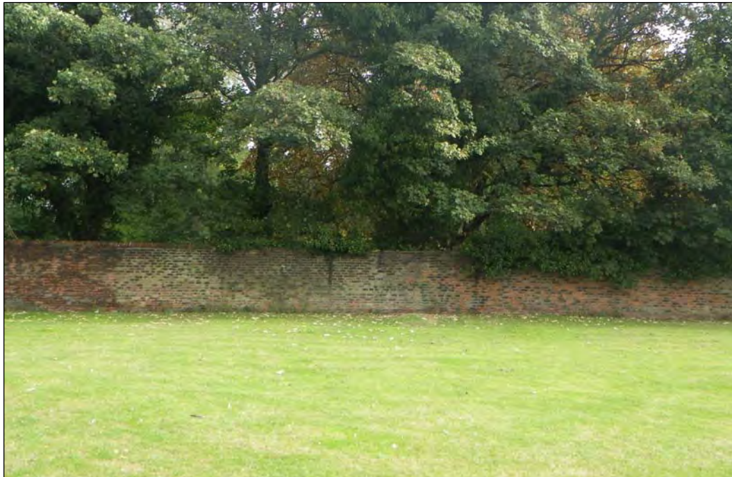
Plate 6: The distempered portion of the west wall. Two metal brackets are visible
