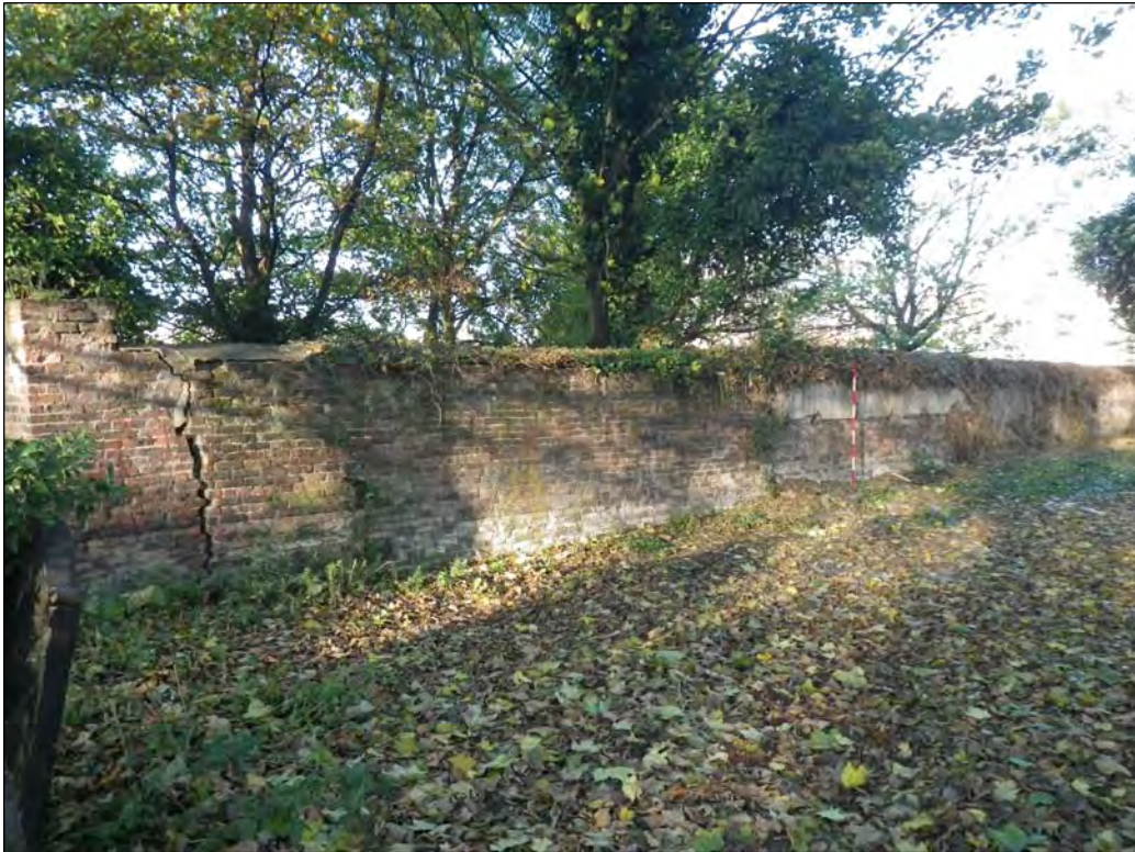
Plate 25: Western part of the gaol-yard wall southern face following removal of vegetation
