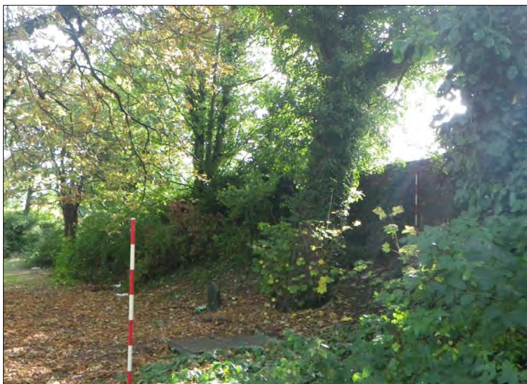
Plate 10: The west wall and the bank to the east of it viewed from within the burial ground, looking south-west. The scale in the background is positioned against the wall's only buttress (2m scales)
