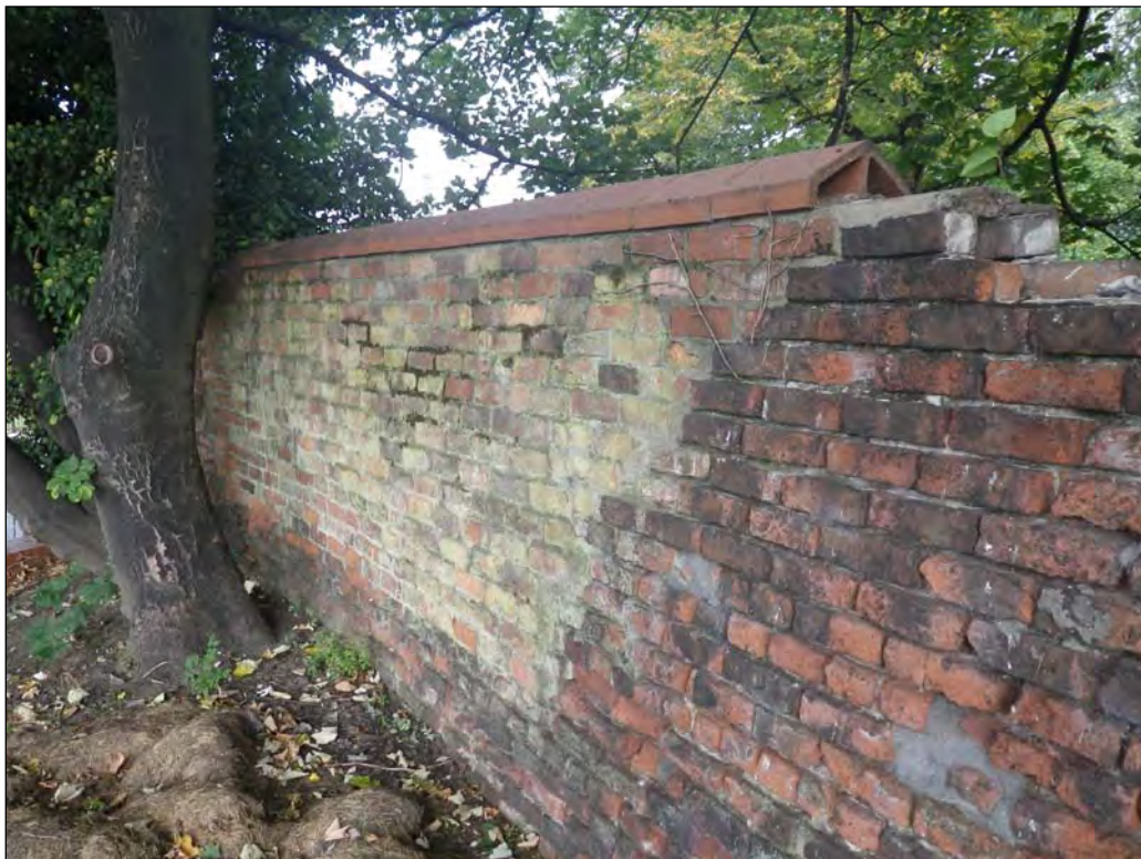
Plate 8: Later rebuild of the northernmost part of the west wall with modern coping
