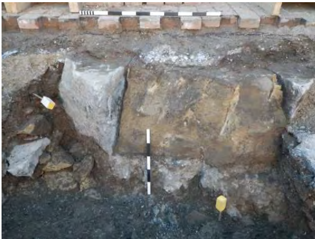
Plate 5: Late nineteenth-century reconstruction of the dock upper stonework sat on concrete; looking south-west
