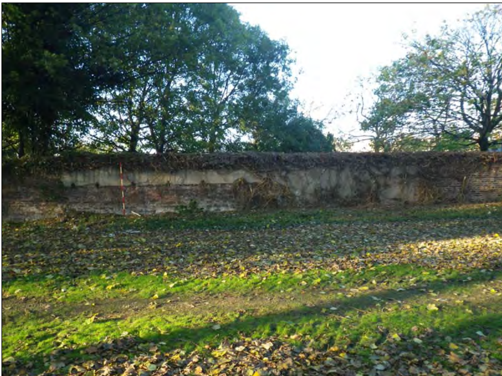
Plate 26: Central part of the gaol-yard wall southern face following removal of vegetation
