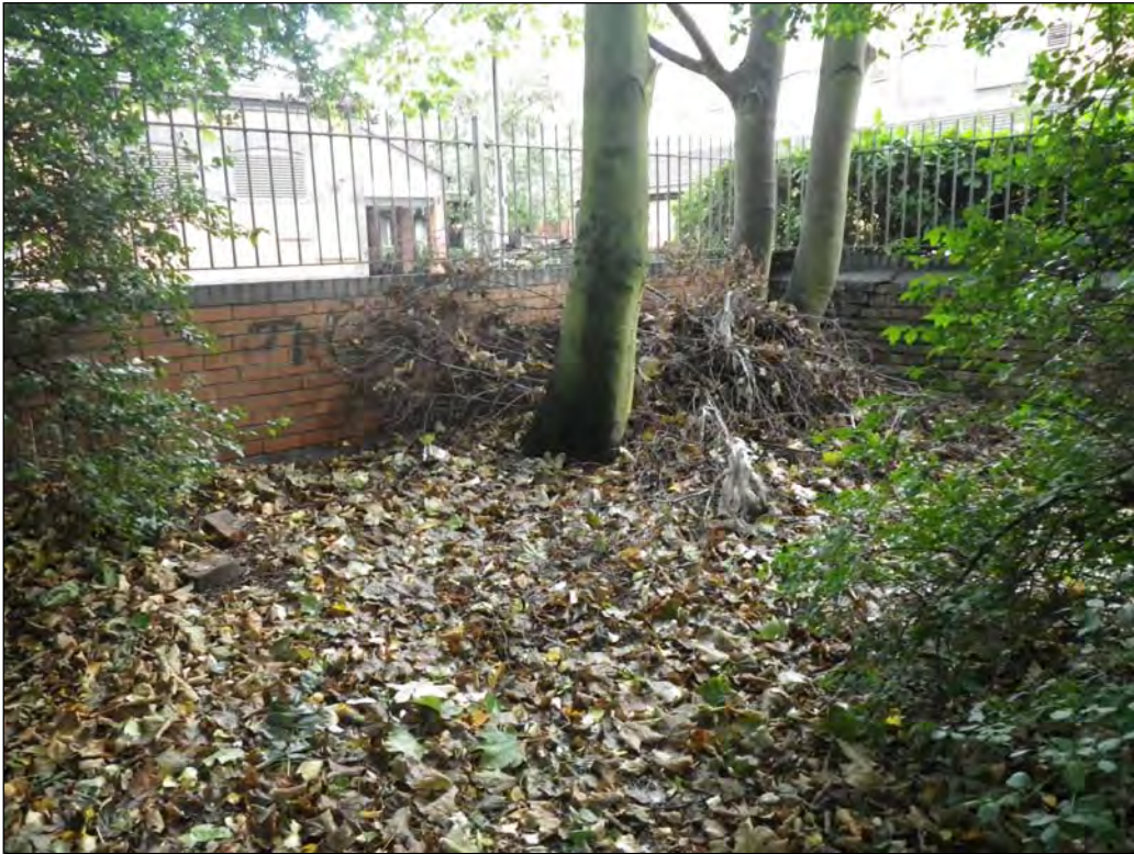
Plate 43: View of the south-east corner of the burial ground showing how the build-up of soil and litter has completely obscured the original wall
